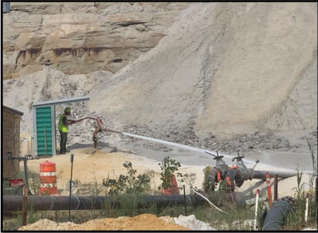
Figure 13.4 - Hydraulic mining utilizing a monitor to produce silica sand slurry for pumping to the processing plant.
