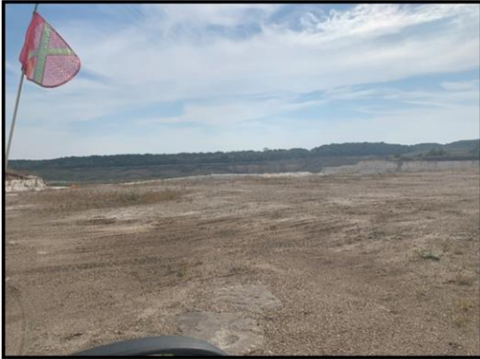
Figure 13.2 - A bench of St. Peter sandstone after clearing and grubbing has prepared the sandstone for drilling and blasting.
